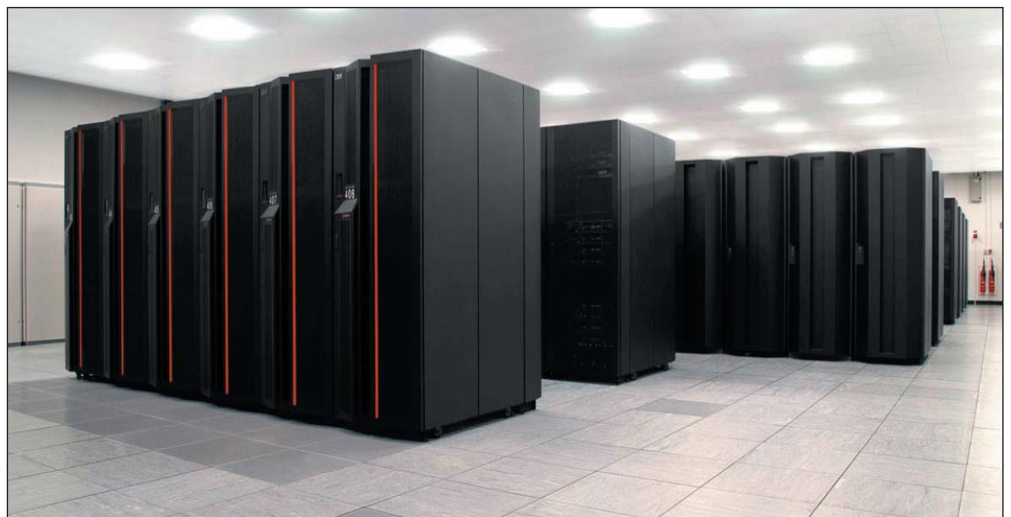
The UK's Engineering and Physical Sciences Research Council, EPSRC, recently agreed that 5% of HPCx resources should be donated to DEISA.
